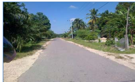
Gambar 1. Jalan Aspal (Survei Lapangan, 2017)
